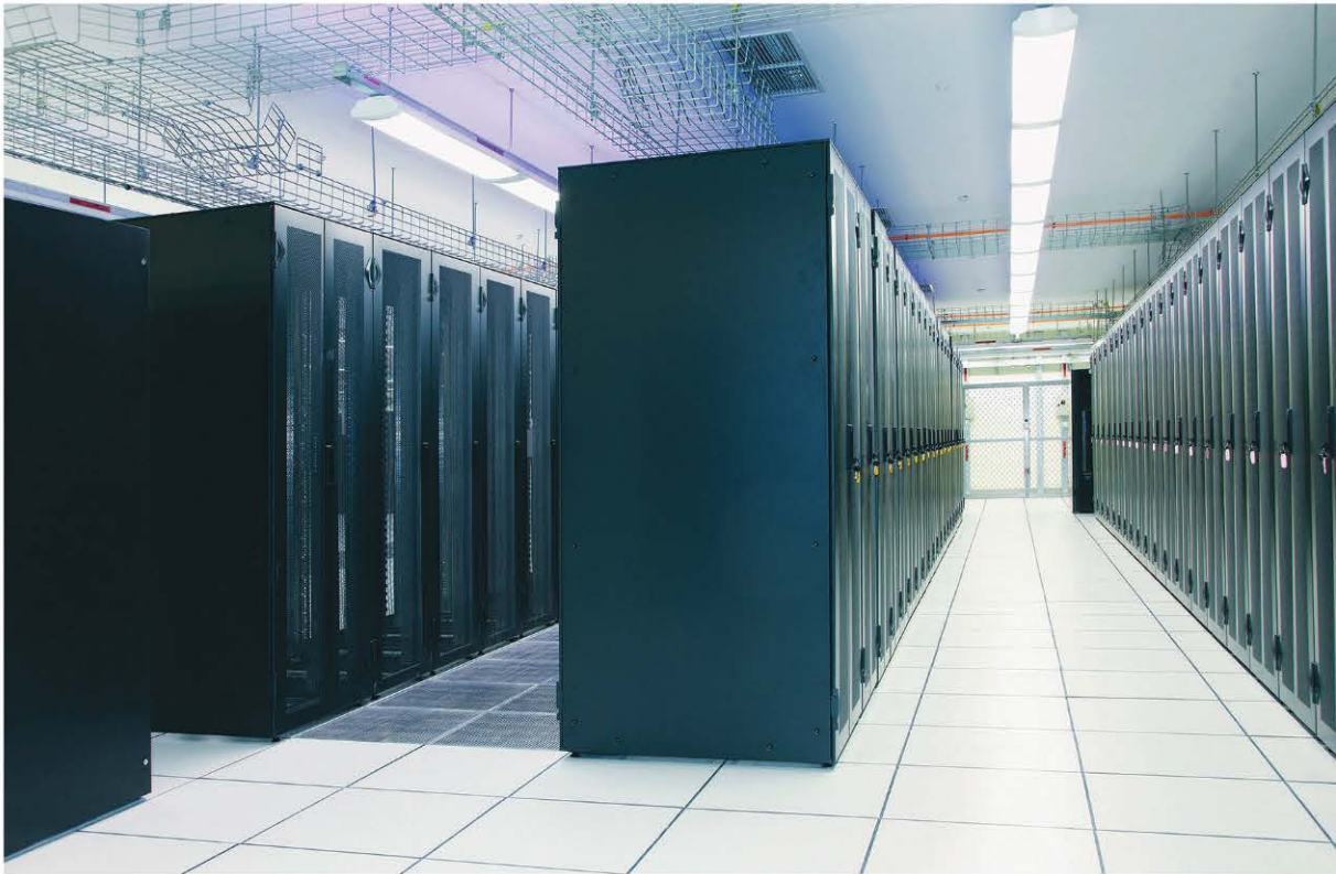
↑ The 87,000-square-foot data centre in Techno Park was built at a cost of $85 million
